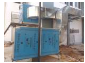
AHU (AIR HANDLING UNIT) (FRESH & EXHAUST)
